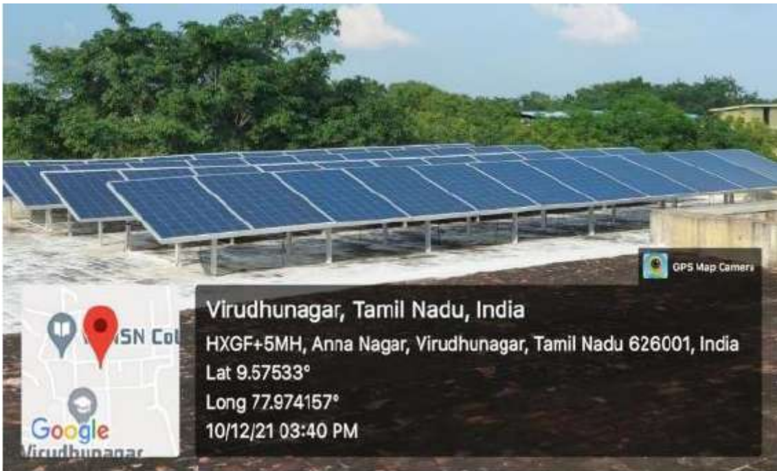
Solar Panel at Arts Block
