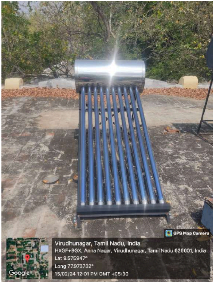
Solar Water Heater at Science Block
