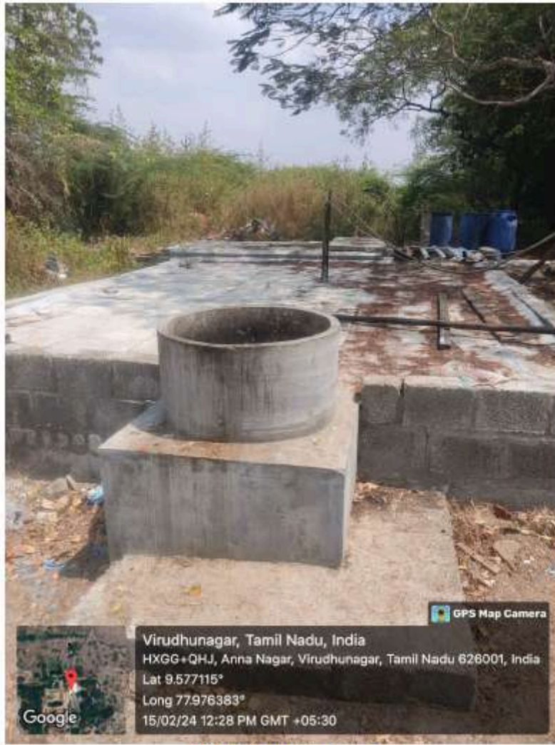
Bio Gas Plant At Boys Hostel
